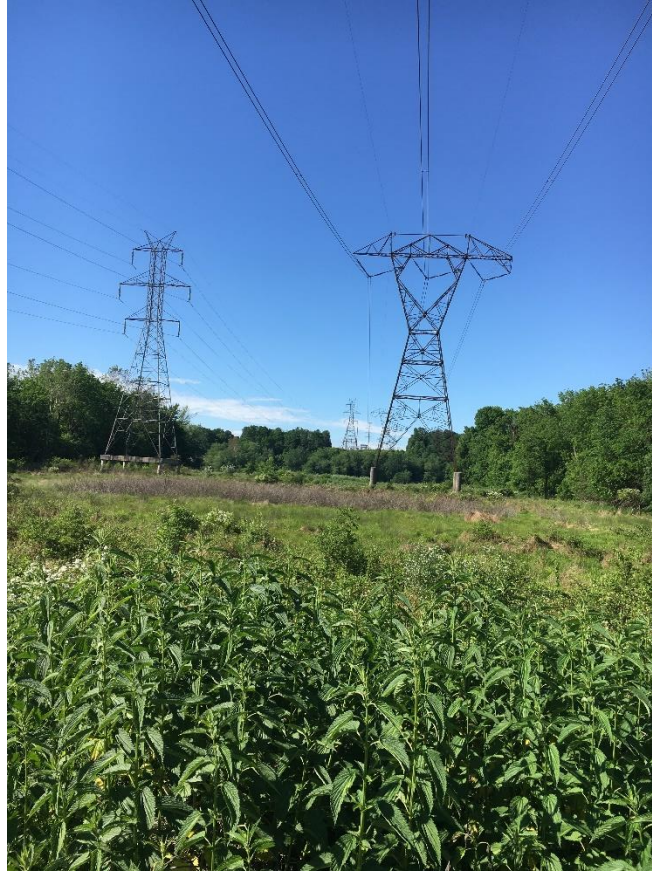
Figure 63 – Electrical distribution ‘power’ lines near the C&O Canal in Maryland. (Credit: Sten Odenwald).
